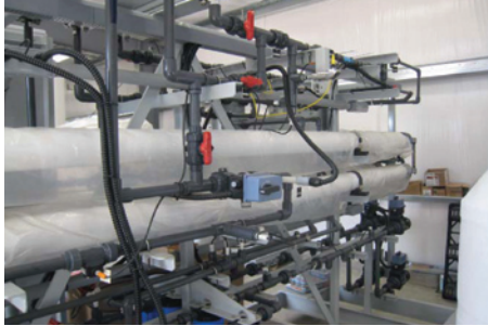
Reverse osmosis system
