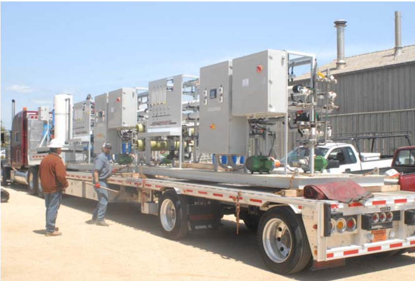
Figure 10. RO skids and instrument control panels.
