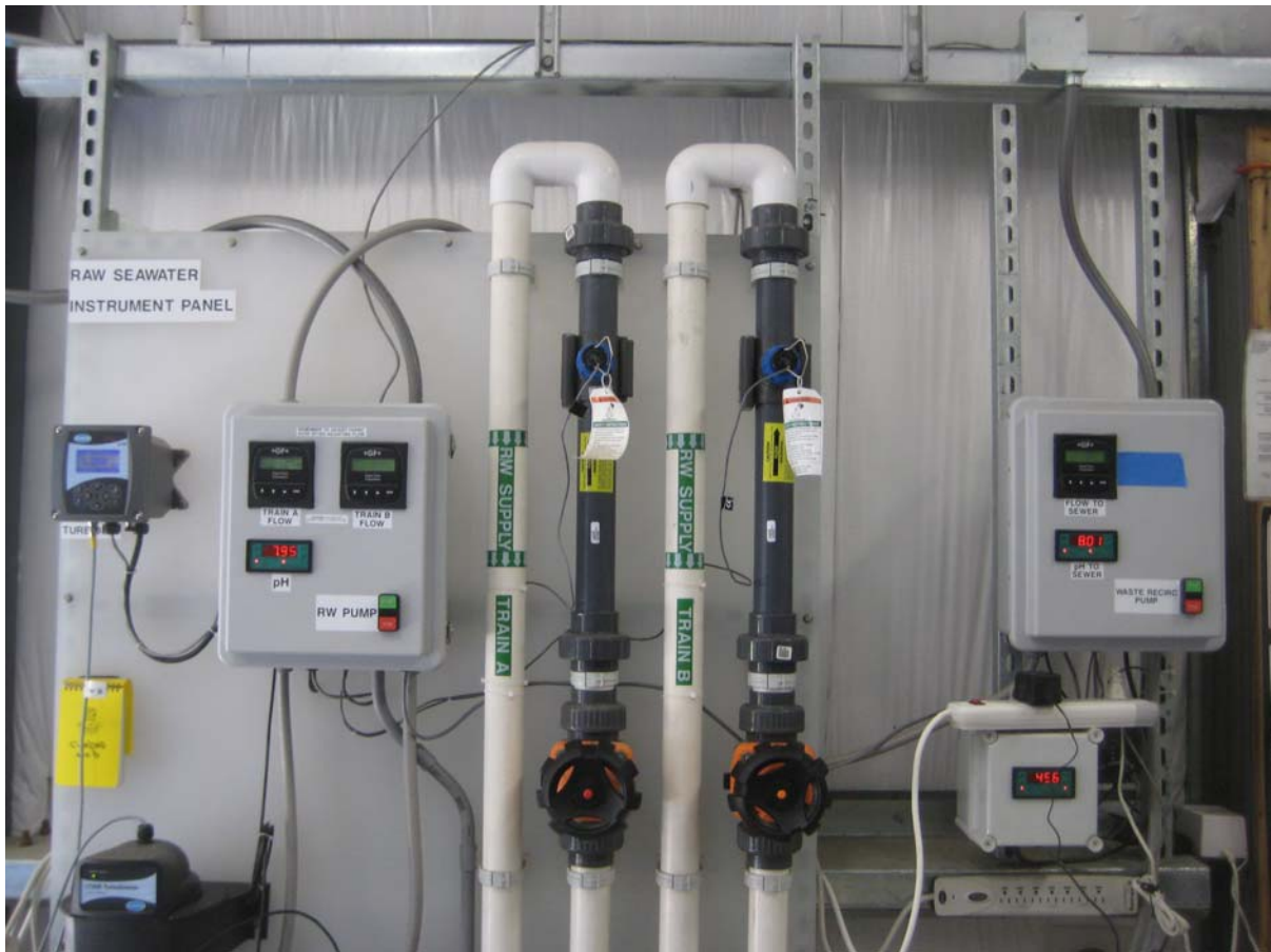
Figure 11. Raw seawater instrument panel.
