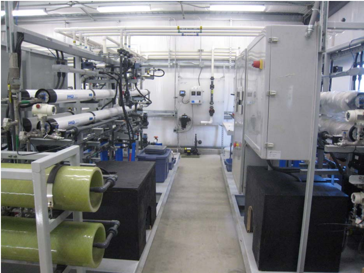
Figure 4. Seawater reverse osmosis skids. Two skids, each with two RO trains, allowed testing of different RO membranes and configurations.
