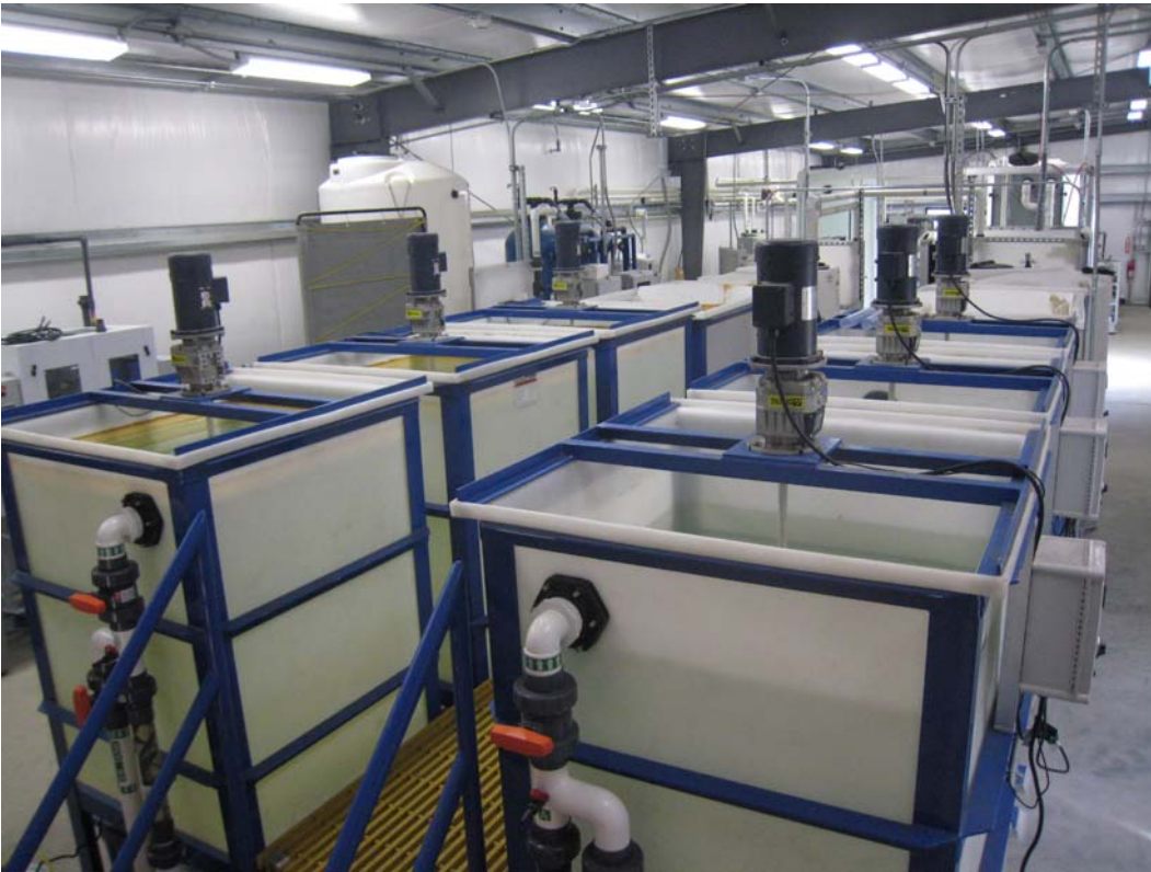
Figure 5. Pretreatment system flocculation and sedimentation basins.
