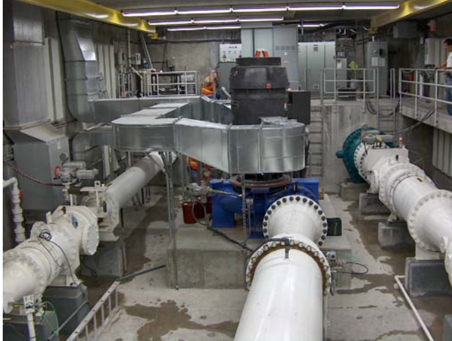
Figure 6: Example Micro-hydro Installation
