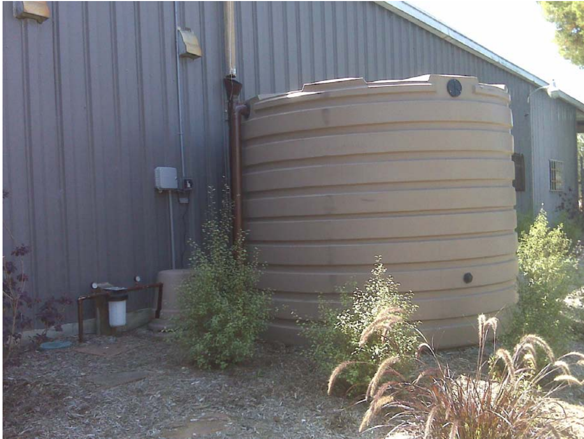
Figure 1: Rainwater Storage Tank at SqCWD Headquarters Office ( ~2,000 gallons)
