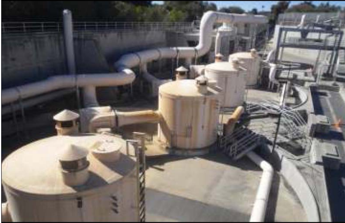
Figure 2: Trickle Filter Odor Scrubbers
