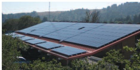
Solar panels at the City of Santa Cruz Graham Hill Water Treatment Plant.
