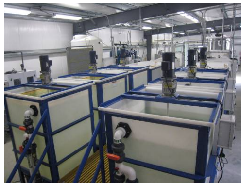
Pilot Horizontal Flocculation Mixing Basins
