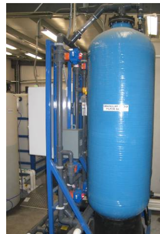
Pilot Pressurized Granular Media Filters
