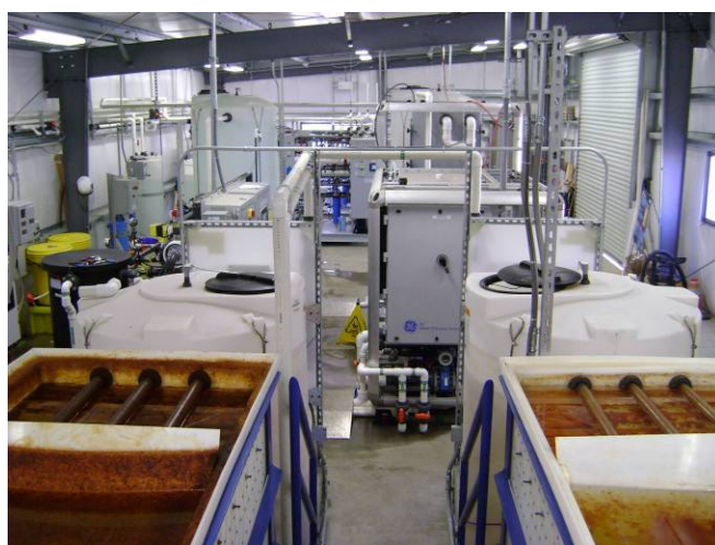
Equipment Installed in the Pilot Plant Building
