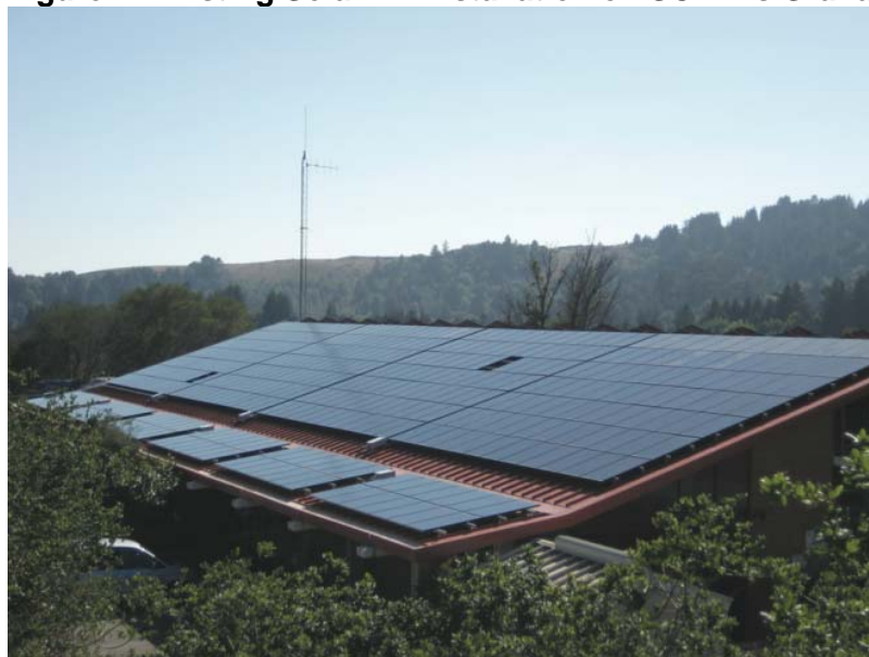
Figure 1: Existing Solar PV Installation on SCWD's Graham Hill WTP
